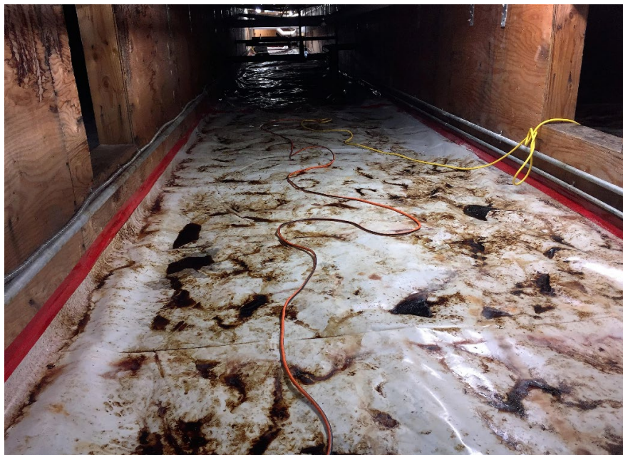
Water damage under subflooring/ crawlspace
